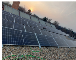
Flansch-Tech Kft. | 113,25 kWp
